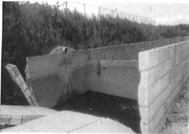
Figure 10: Stagnant water, a breeding site for mosquitoes.
