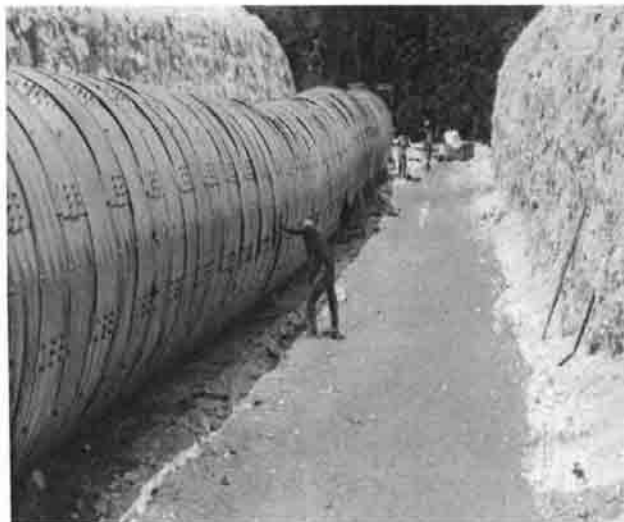
Figure 6: CPS drain pipe being installed at a low point along the alignment.
