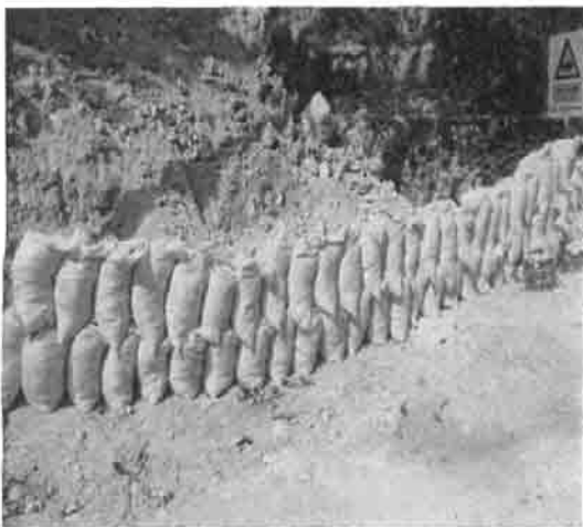
Figure 2: Showing sand bags placed at K 61 + 500 to prevent erosion of marly earth material into adjacent drain and onto the public thoroughfare.
