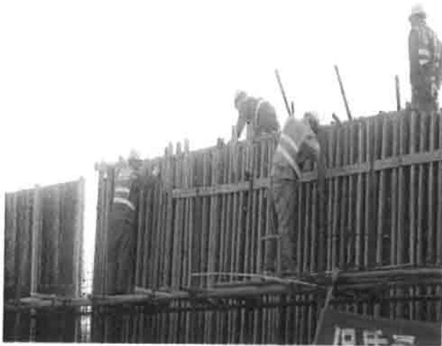
Figure 9: Workers at height without wearing any harness at box culvert construction site at about K 56 +.
