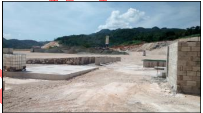
Photo 5: Construction of the aggregate stabilization plant in progress at K52. (Photo taken by Environmental Officer, NEPA on 16 January 2015)
