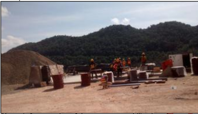
Photo 4: Construction of the aggregate stabilization plant in progress at K52. (Photo taken by Environmental Officer, NEPA on 16 January 2015)
