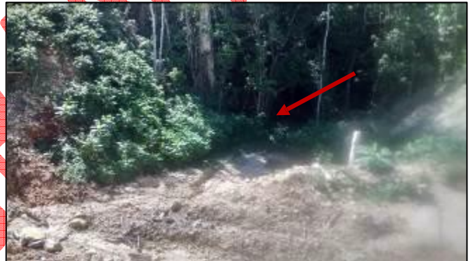
Photo 4: Sinkhole around K62+600 (Photo taken by Environmental Officer, NEPA on 7 November 2014)
