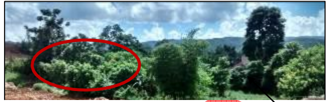
Photo 6: Soakaway under construction. (Encircled in red) (Photo taken by Environmental Officer, NEPA on 7 November 2014)
