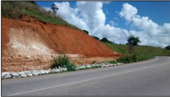
Photo 1: Sandbags around K46+800 at the roundabout where section 3 begins. (Photo taken by Environmental Officer, NEPA on 7 November 2014)
