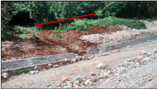
Photo 3: Sinkhole around k48+900 encircled in red. (Photo taken by Environmental Officer, NEPA on 7 November 2014)
