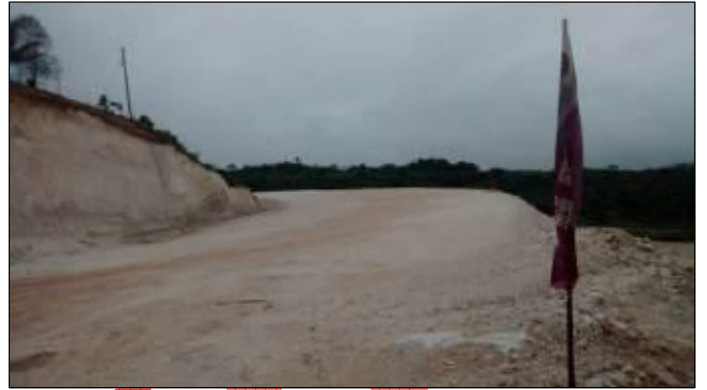
Photo 2: Section of the alignment around K54 ready to be paved. (Photo taken by Environmental Officer, NEPA on 7 November 2014)
