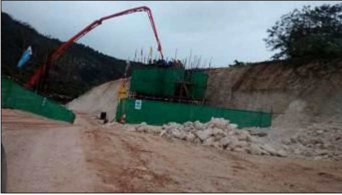
Photo 1: Bridge construction at K50 (Photo taken by Environmental Officer, NEPA on 7 November 2014)
