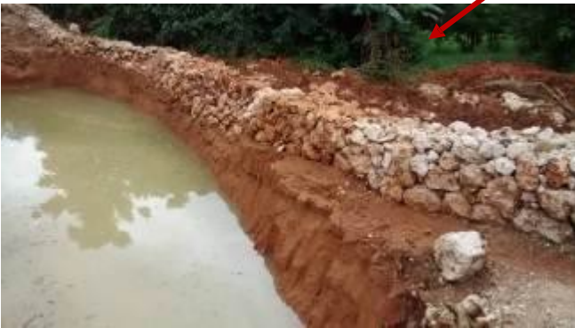
Photo 3: Holding pond around K 47+080 to prevent storm water runoff into private property. (Photo taken by Environmental Officer, NEPA on 7 November 2014)
