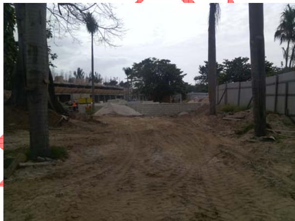
Photo 4: Work underway on the erection of the main building. Photo taken 29 January 2016 by NEPA Officer.
