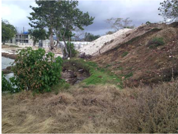
Photo 7: Stockpiles of soil and marl at the water's edge, without any berm or covering. Photo taken 29 January 2016 by NEPA Officer
