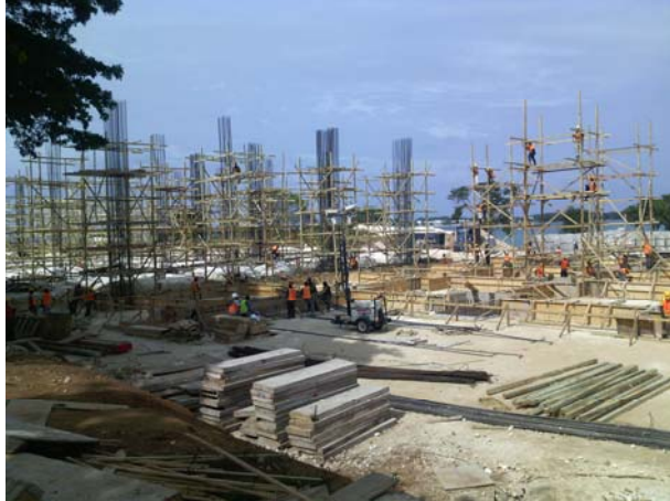
Photo 1: Work underway on the erection of the main building. Photo taken 29 January 2016 by NEPA Officer.
