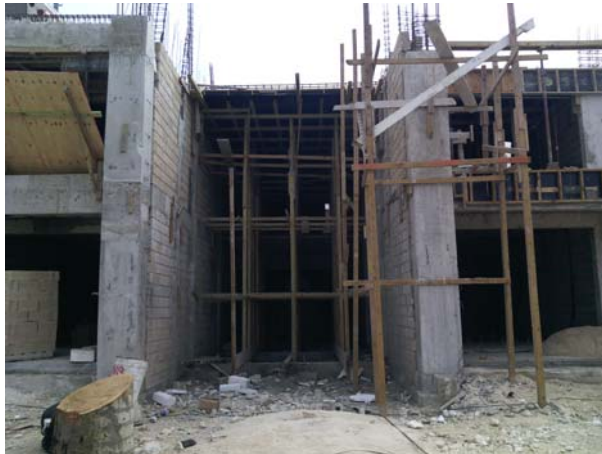
Photo 3: The structure occupying the proposed break between buildings 1 and 2. Work underway on the erection of the main building. Photo taken 29 January 2016 by NEPA Officer.
