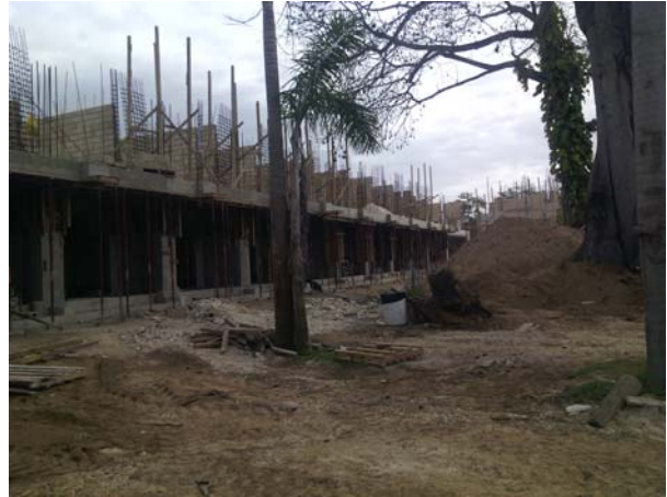
Photo 2: A view of the stage of construction of building 1, under construction contrary to the approved drawings. Photo taken 29 January 2016 by NEPA Officer.
