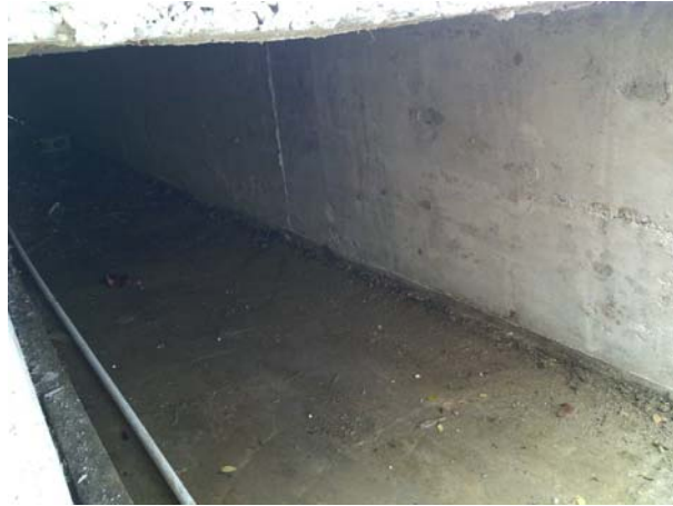
Photo 8: Inside the box culvert leading to the marine environment. Note there were no sediment traps inside the drain. Photo taken 29 January 2016 by NEPA Officer
